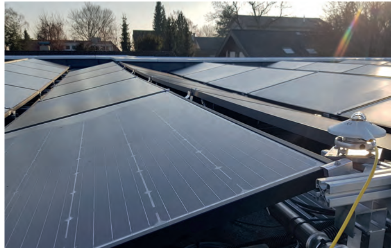
Demonstration system with a PVT collector array.
