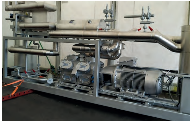
Butane high temperature heat pump manufactured by Johnson Controls.
